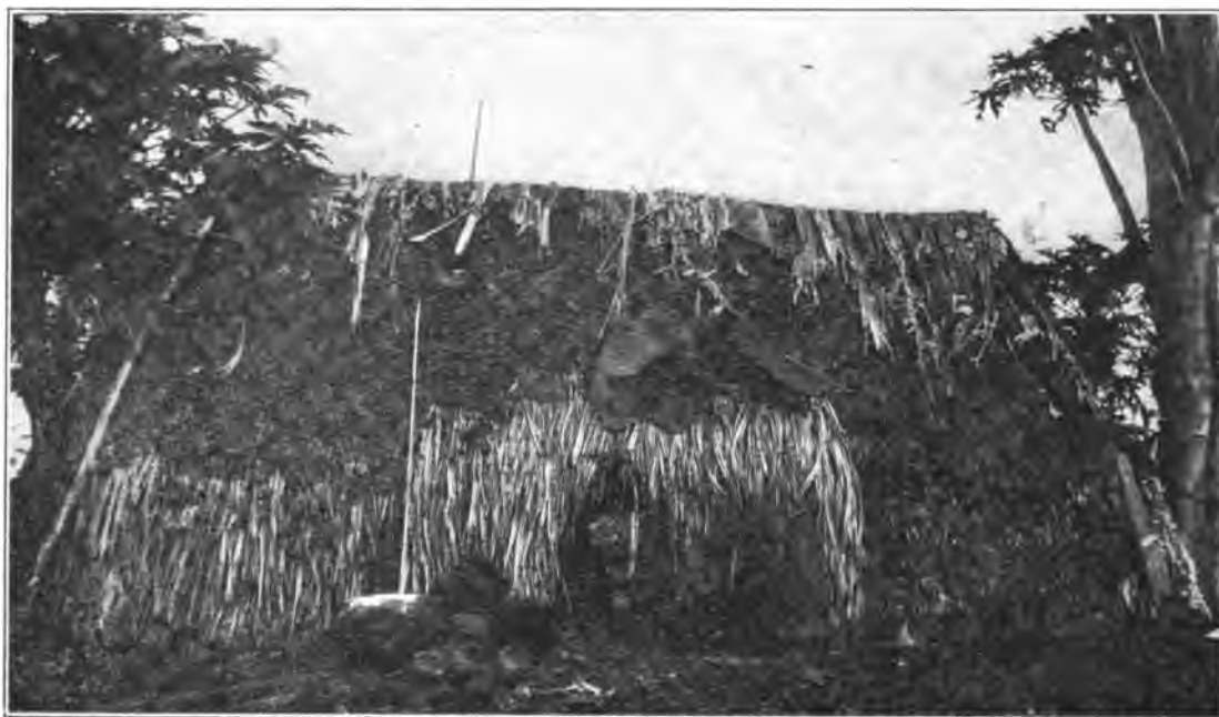
FIG. 83. HOUSE NEAR HILO NEEDING A NEW ROOF.
